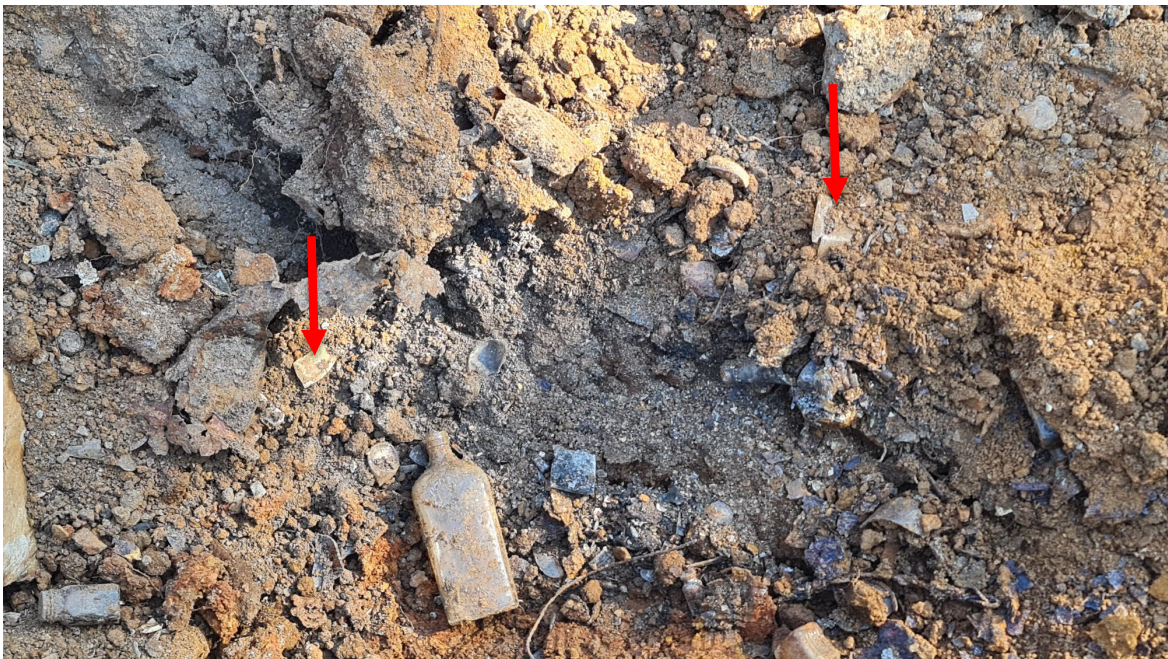
Sandy clay fill soil in former tennis court area containing metal, glass and pieces of asbestos cement sheet debris. Arrows indicates asbestos cement sheet debris
