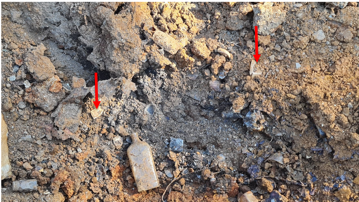
Fill soil in former tennis court area containing metal, glass and pieces of asbestos cement sheet debris. Arrows indicates asbestos cement sheet debris
