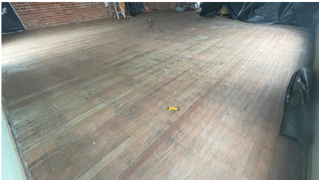
Timber floor in the large rear room in the St Augustines building at St John of God Richmond Hospital, 177 Grose Vale Road, North Richmond NSW at completion of visual clearance inspection on 23 September 2022
