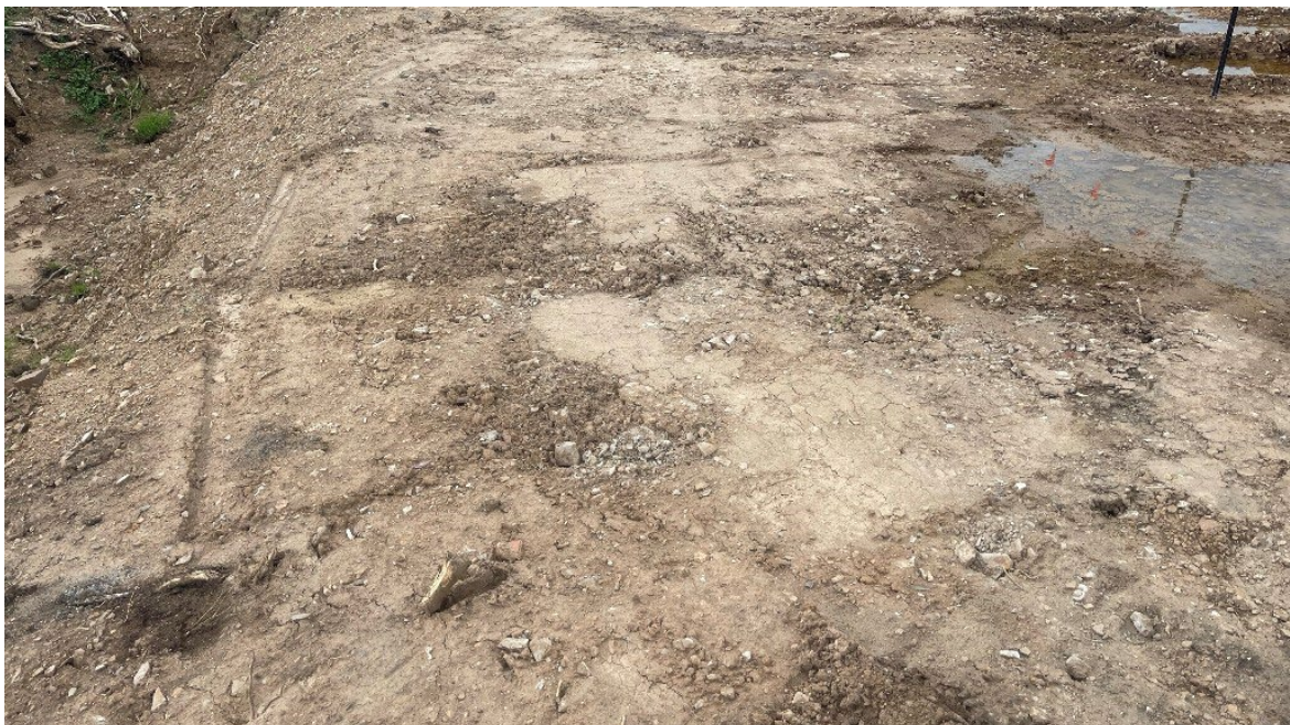
Base of the excavated area at the rear of the former Monastery Building on 27 October 2022 at the completion of the removal of asbestos contaminated fill soil
