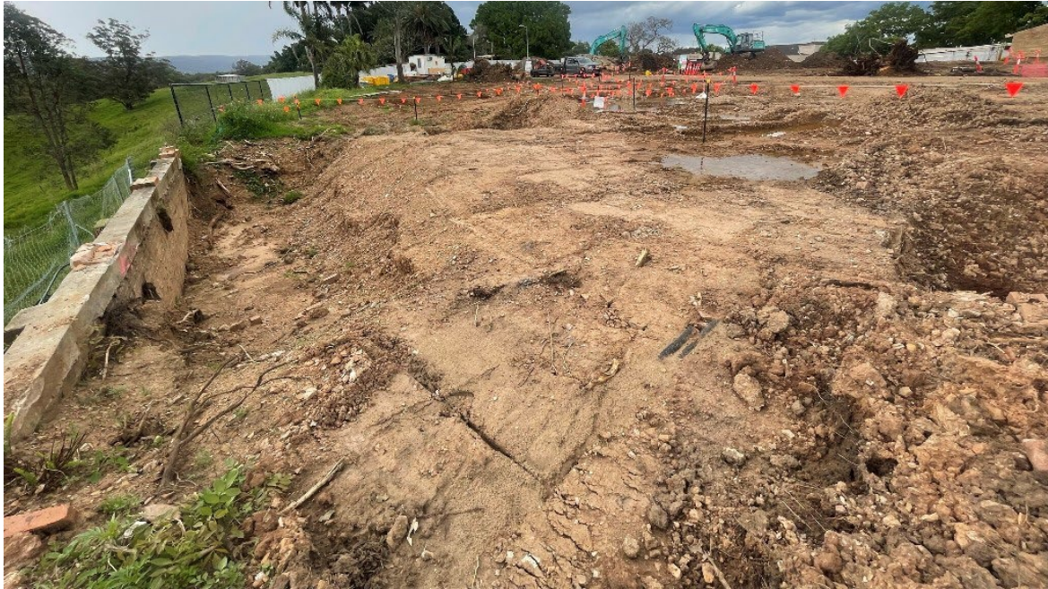
Excavated area at the rear of the former Monastery Building on 27 October 2022 at the completion of the removal of asbestos contaminated fill soil
