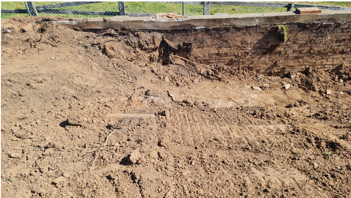
Brick retaining wall at the rear of the former Monastery Building. Fill removed from the area where the wall is exposed and fill soil remaining against the wall contains fragments of asbestos cement sheet debris
