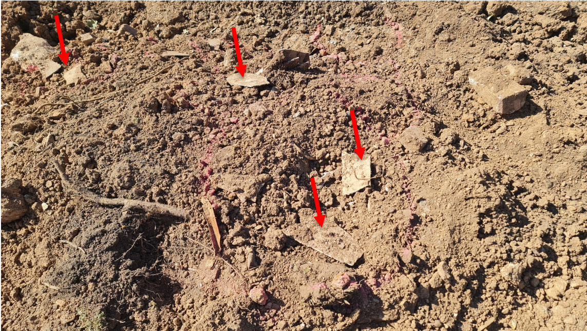
Asbestos cement sheet debris in fill soil located behind the retaining wall at the rear of the former Monastery Building
