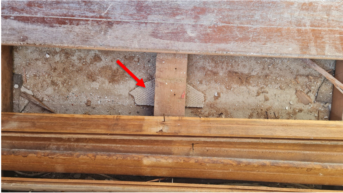
Asbestos cement packing piece between timber floor joist and concrete floor in the upper level of the Monastery Building. This material contains chrysotile asbestos and amosite asbestos
