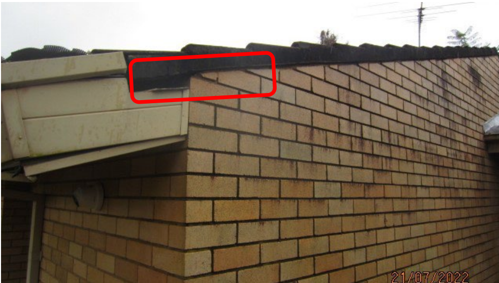
Photograph No. 9: Asbestos cement sheet supporting strip below verge tiles and upper eave / anti-ponding board below lowest row of roof tiles on the Consulting Rooms building
