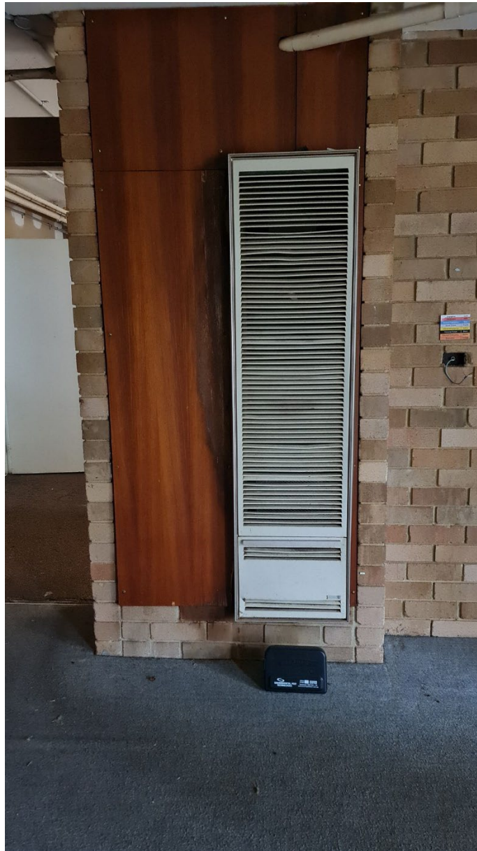
Photograph No. 7: Gas room heater in gymnasium in the lower level of the CTC Building. The flue attached to this heater is moulded asbestos cement
