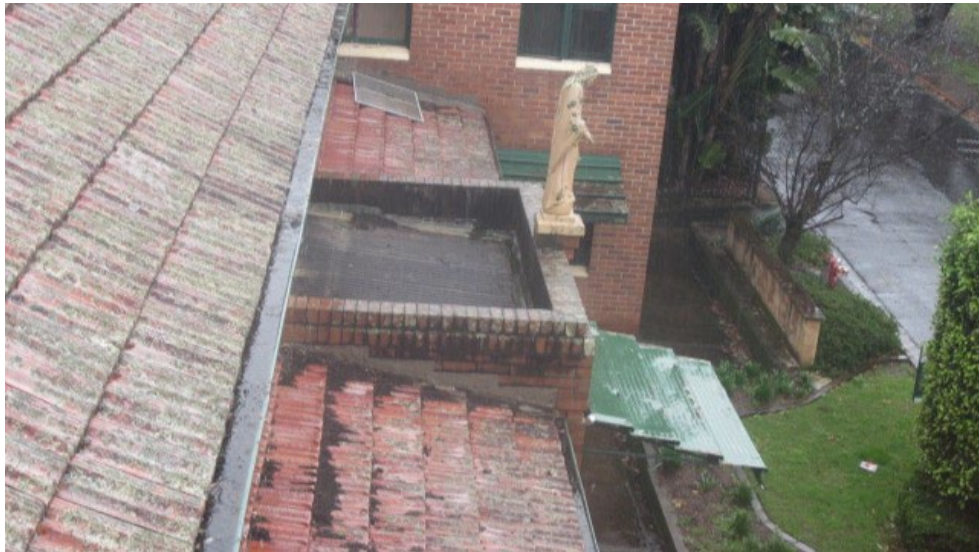
Photograph No. 10: Corrugated asbestos cement sheet roof cladding over front entry area to the Monastery building
