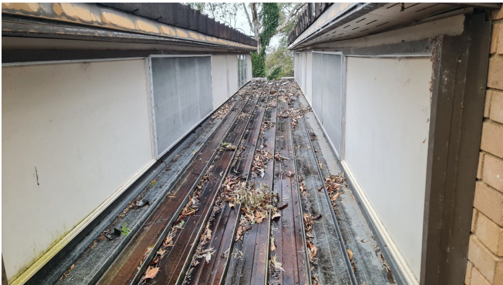
Photograph No. 2: Flat asbestos cement sheet infill panels and eave lining in the centre roof area of the CTC Building
