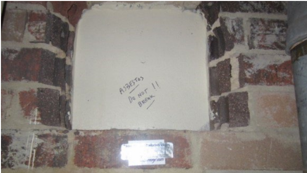
Photograph No. 6: Rear side of typical asbestos free fibrous cement sheet infill panel on plumbing duct in typical bathroom in CTC Building. A sample of this material was analysed and found to be free of asbestos
