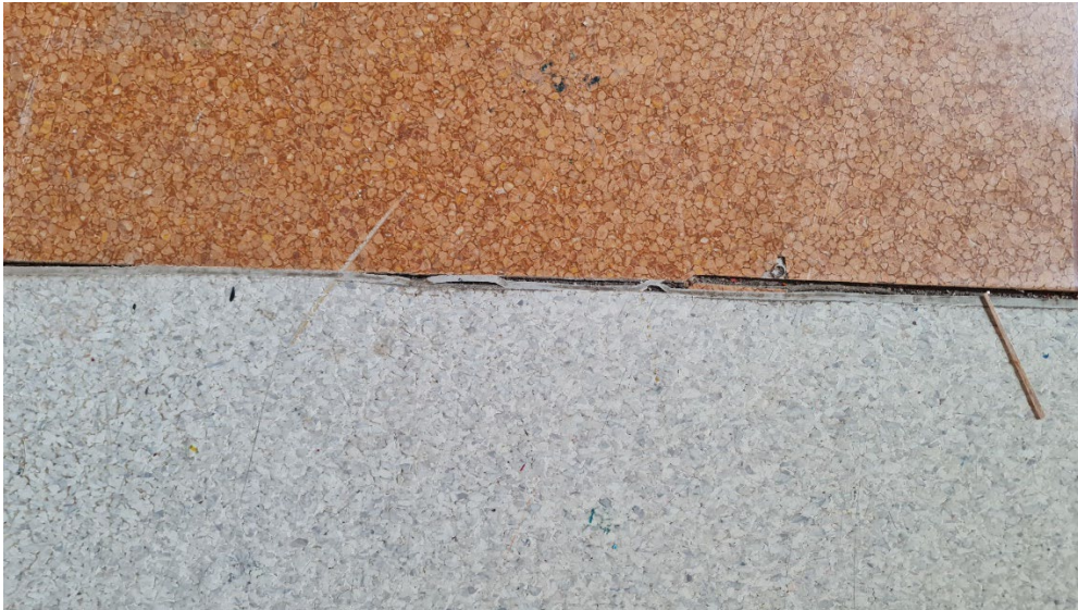
Photograph No. 12: Orange / brown coloured sheet vinyl in rear room of the Arts Building. This vinyl was analysed and found to have asbestos in the fibrous backing layer. This material is classifiable as friable asbestos
