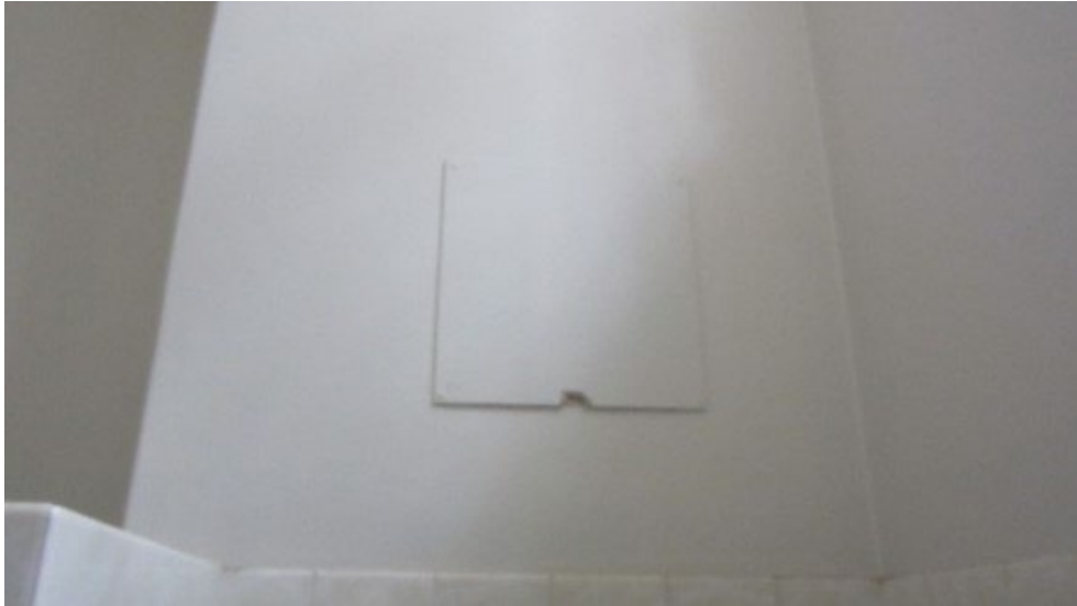
Photograph No. 5: Asbestos free fibrous cement sheet infill panel on plumbing duct in typical bathroom in CTC Building
