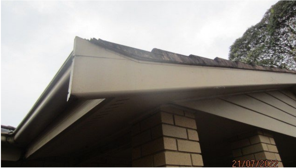
Photograph No. 8: Asbestos free fibrous cement sheet eave lining and verge tile supporting strip on the north west end of the Medical Services building. The gable weatherboard cladding is hardboard 'Weathertex'
