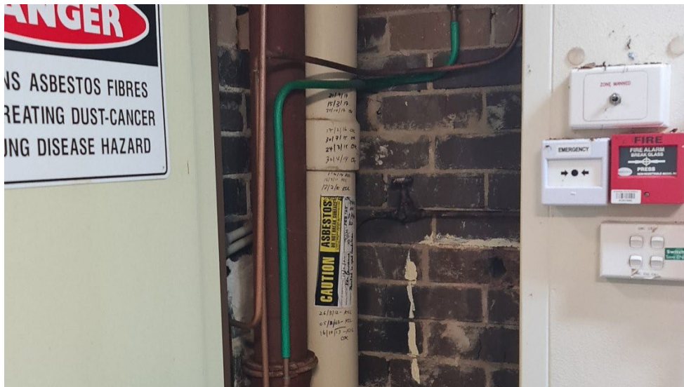
Photograph No. 4: Asbestos cement flue in Duct 6 in CTC Building
