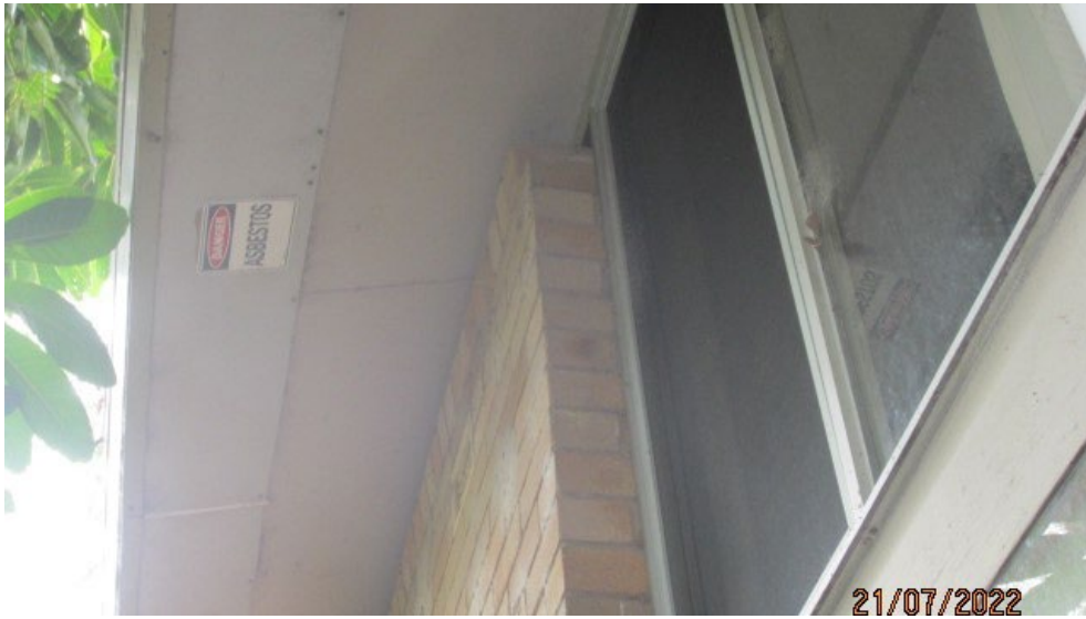
Photograph No. 1: Flat asbestos cement sheet eave lining in the CTC Building
