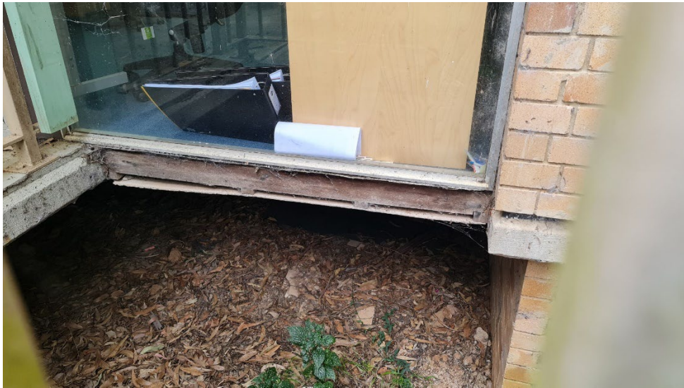
Photograph No. 3: Flat asbestos cement sheet below floor of the St Raphaels unit on the south east side of the CTC Building
