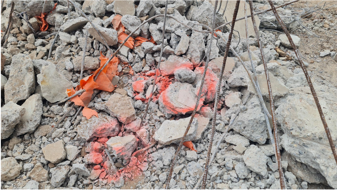
Asbestos cement sheet material embedded on concrete floor slab of the Education Centre building – Contains chrysotile asbestos
