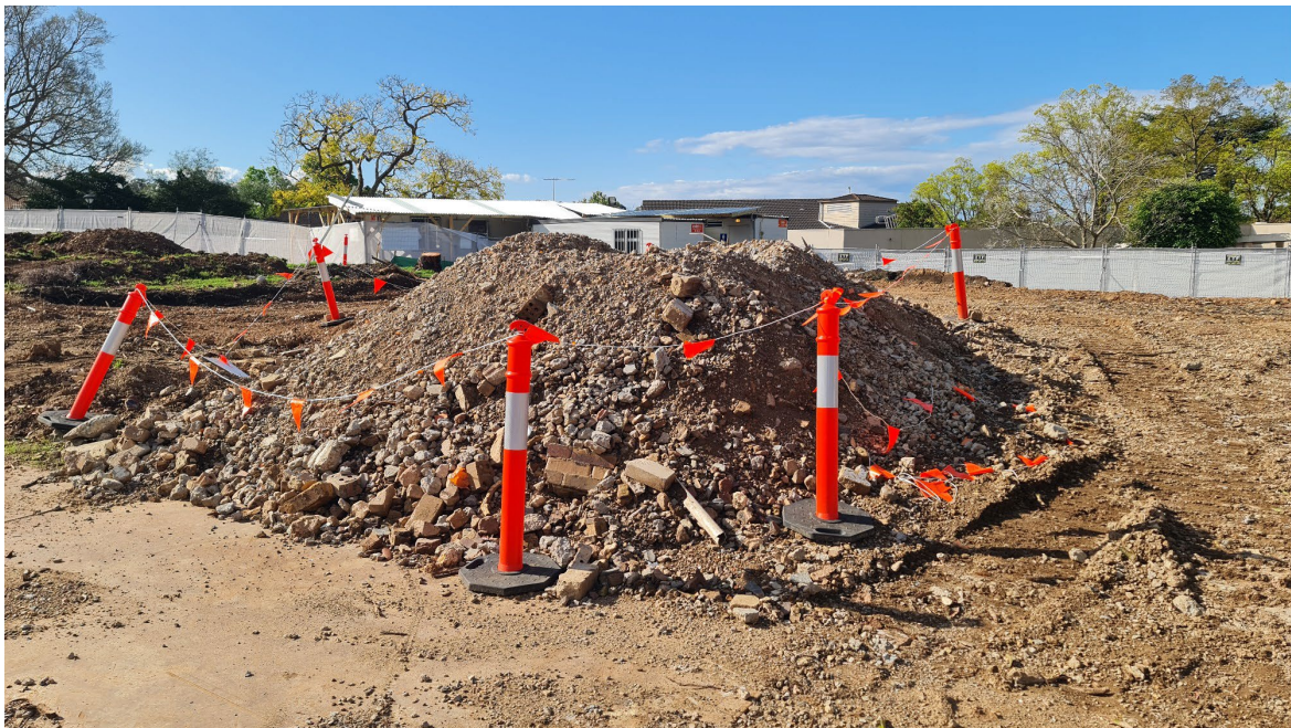
Photograph No. 2: Sandy clay fill soil stockpiled in former chapel building area
