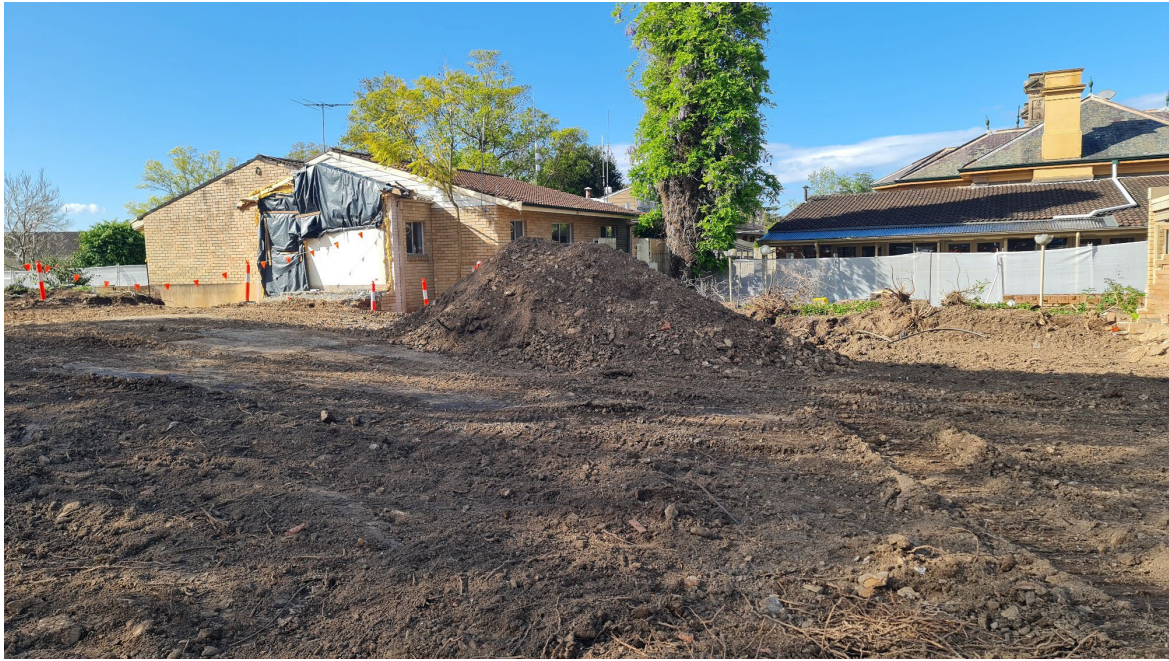
Photograph No. 1: Sandy clay fill soil stockpiled in former medical centre building area
