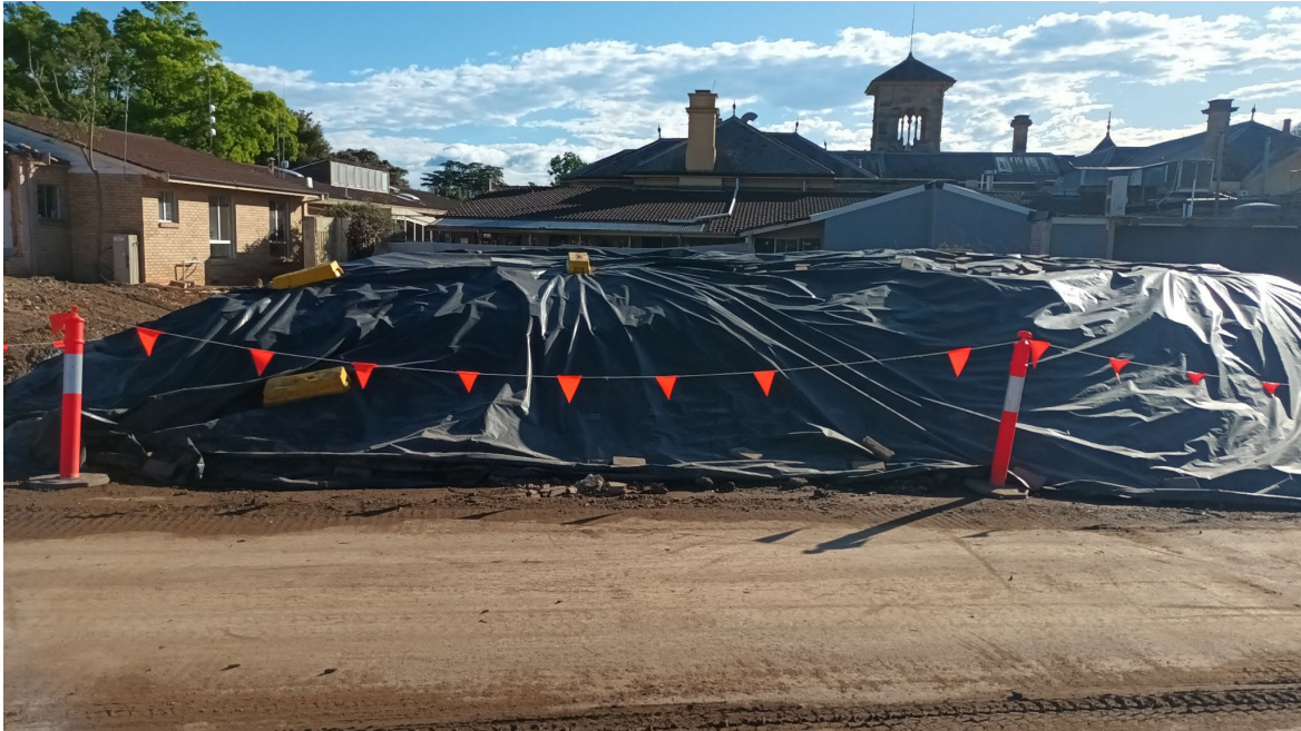
Excavated soil containing asbestos cement sheet debris from the Education Centre area that was stockpiled on 26 October 2022
