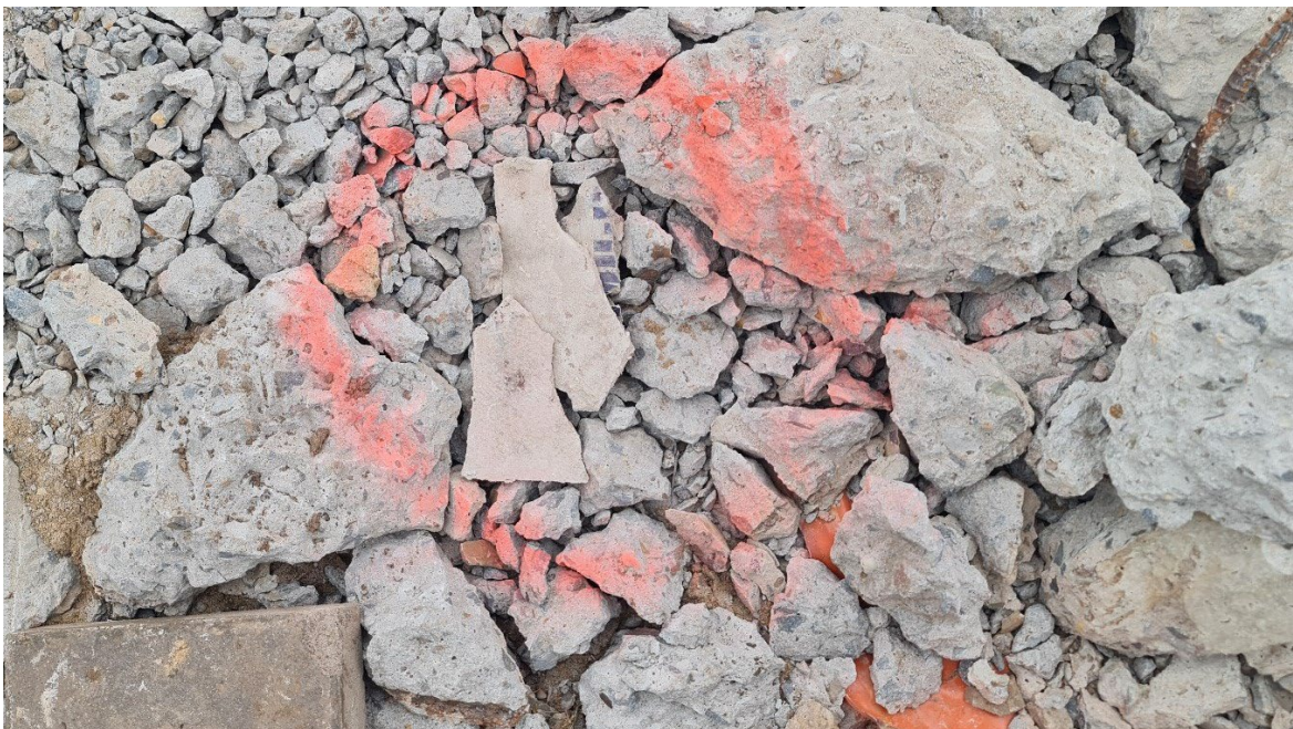
Sample 2 – Asbestos cement sheet material found below concrete floor slab of the Education Centre building – Contains chrysotile asbestos
