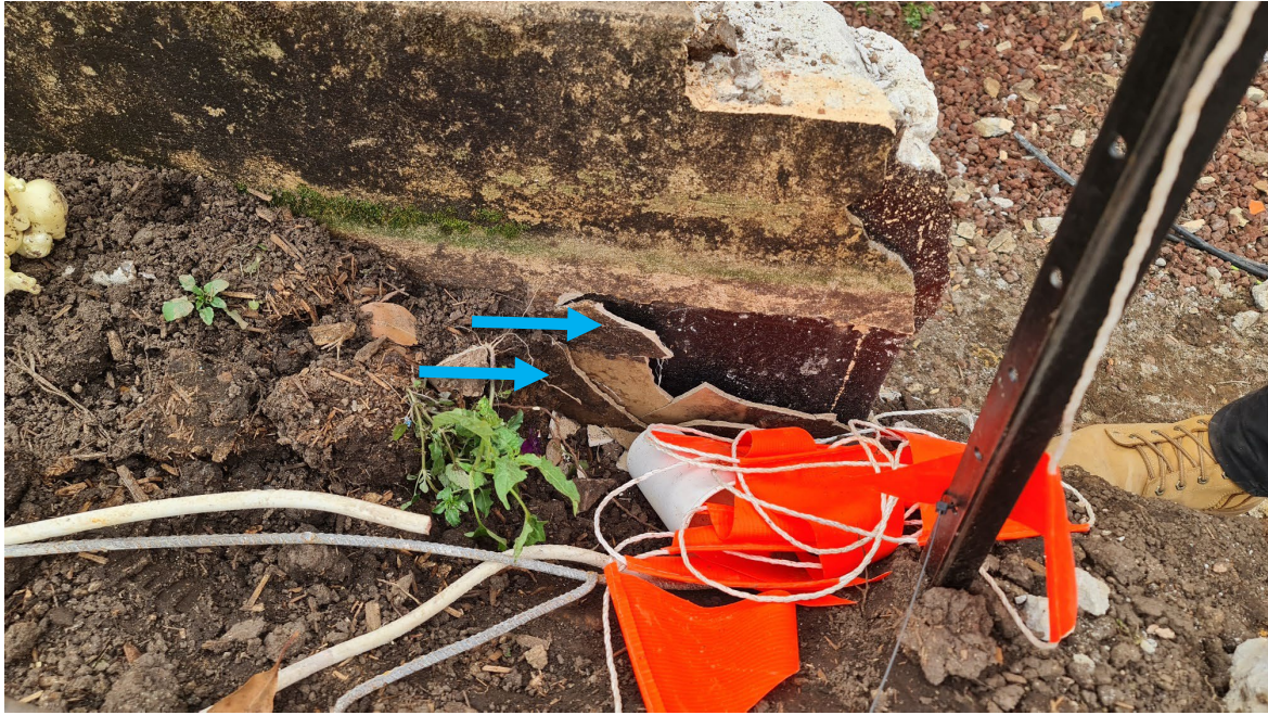
Sample 3 – Two layers of fibrous cement sheet behind retaining wall. A composite sample of these materials was found to be free of asbestos
