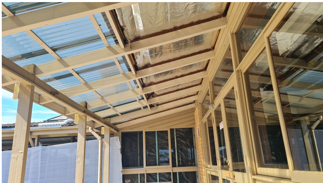
Timber framing in the northern external area in the Food Services Unit at St John of God Richmond Hospital, 177 Grose Vale Road, North Richmond NSW at completion of visual clearance inspection on 19 September 2022
