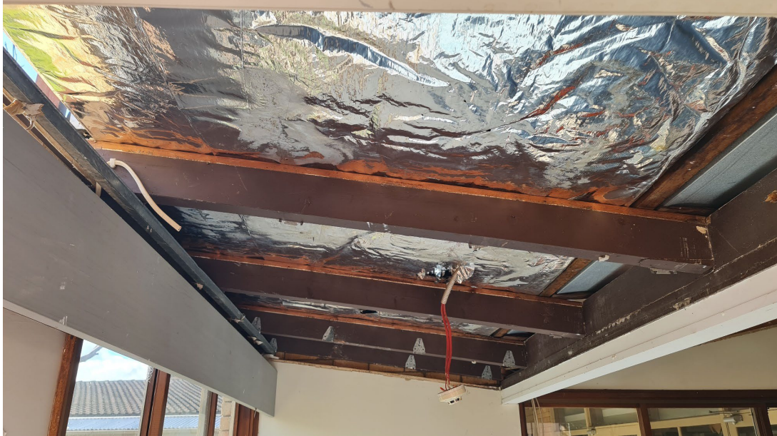
Timber framing in the north west internal area in the Food Services Unit at St John of God Richmond Hospital, 177 Grose Vale Road, North Richmond NSW at completion of visual clearance inspection on 7 September 2022
