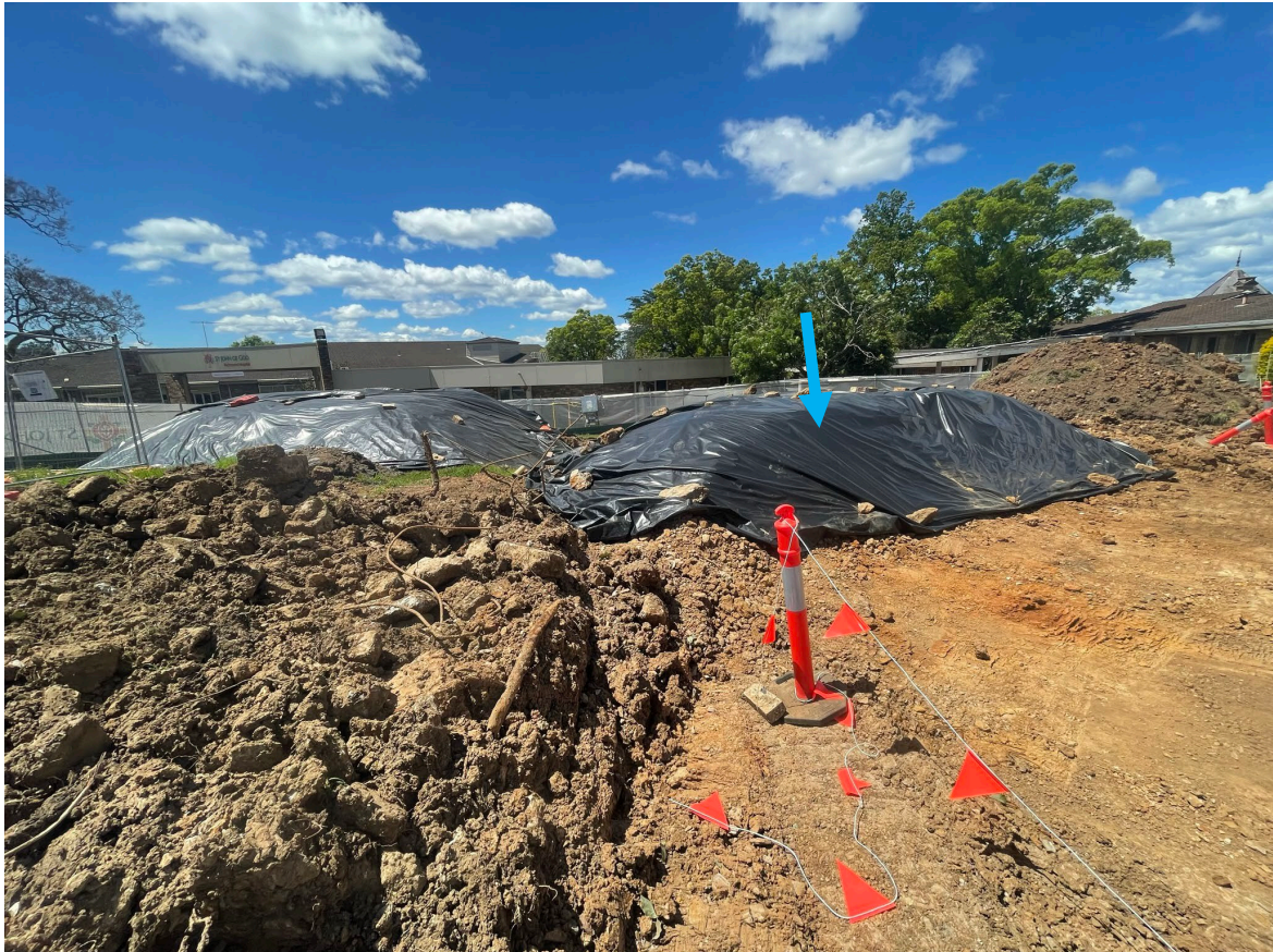
Photograph No. 1: Arrow indicates stockpiled fill soil excavated from across the area on which the former chapel building was located on 2 November 2022
